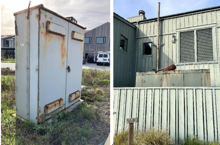
Figure 43 – Examples of environmental corrosion at Coastal Science Campus
