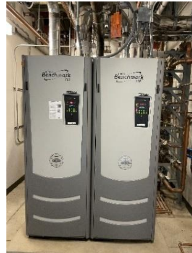
Figure 34 – Existing natural gas boilers
