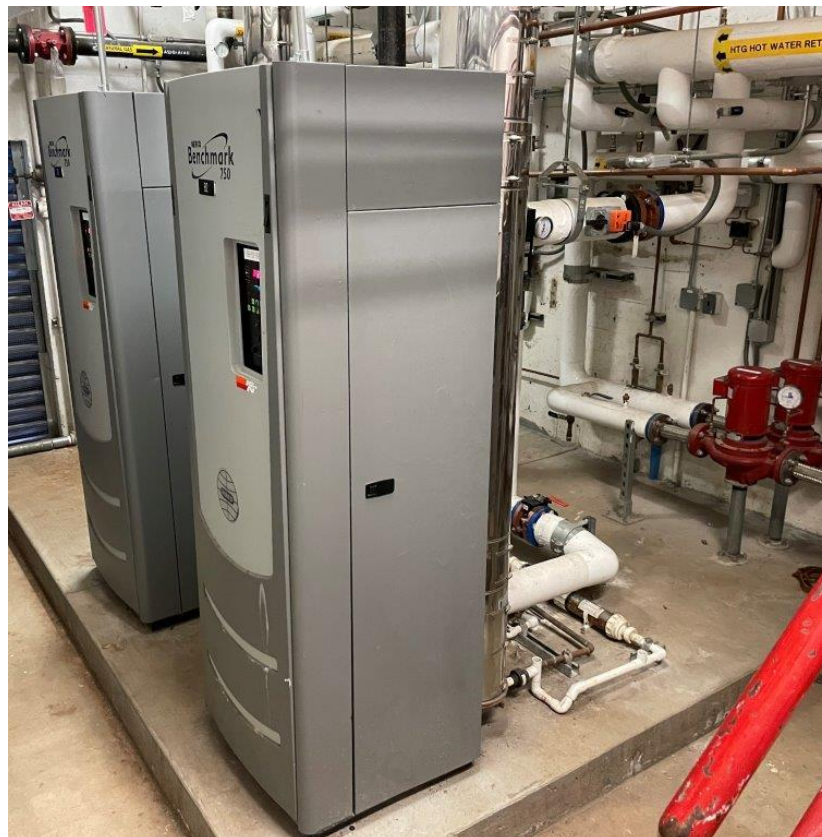
Figure 51 – Gas boilers (good condition)
