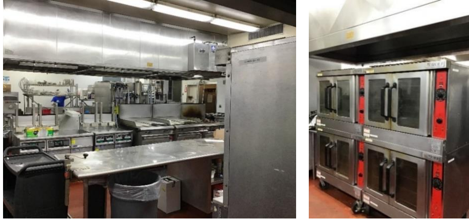
Figure 19 – Existing kitchen equipment
