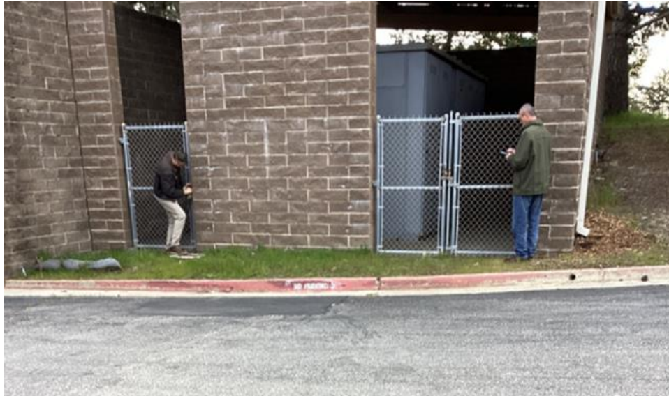
Figure 42 – Enclosed PG&E service at Westside Research Park
