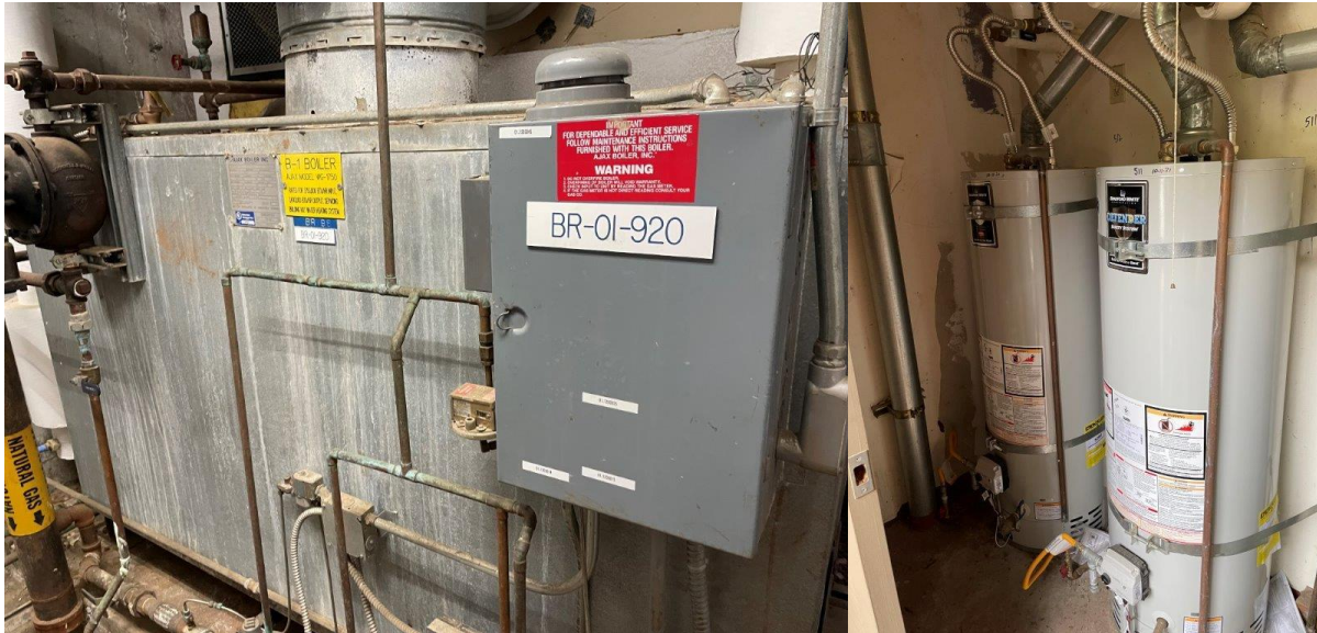
Figure 50 – Existing gas boilers and water heaters
