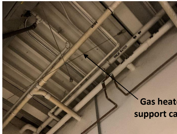
Gas heater support to metal deck
