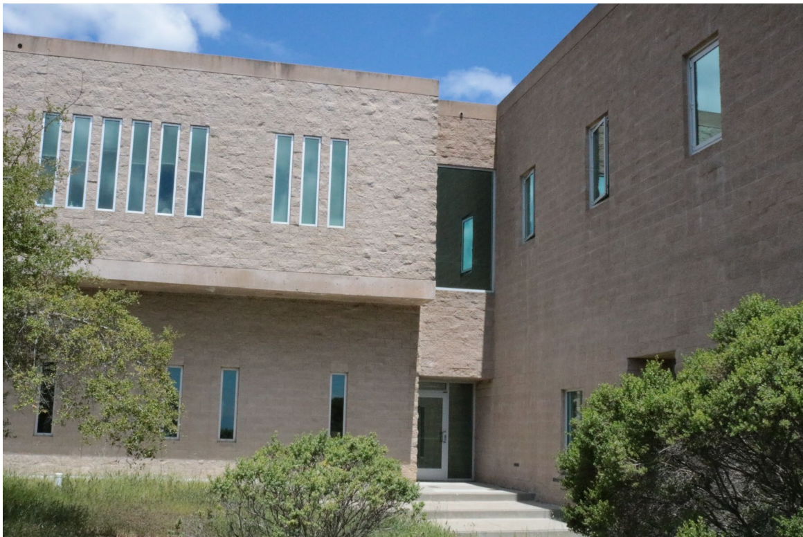
East elevation of Building 3E and south elevation of CAAN 7922, looking north
