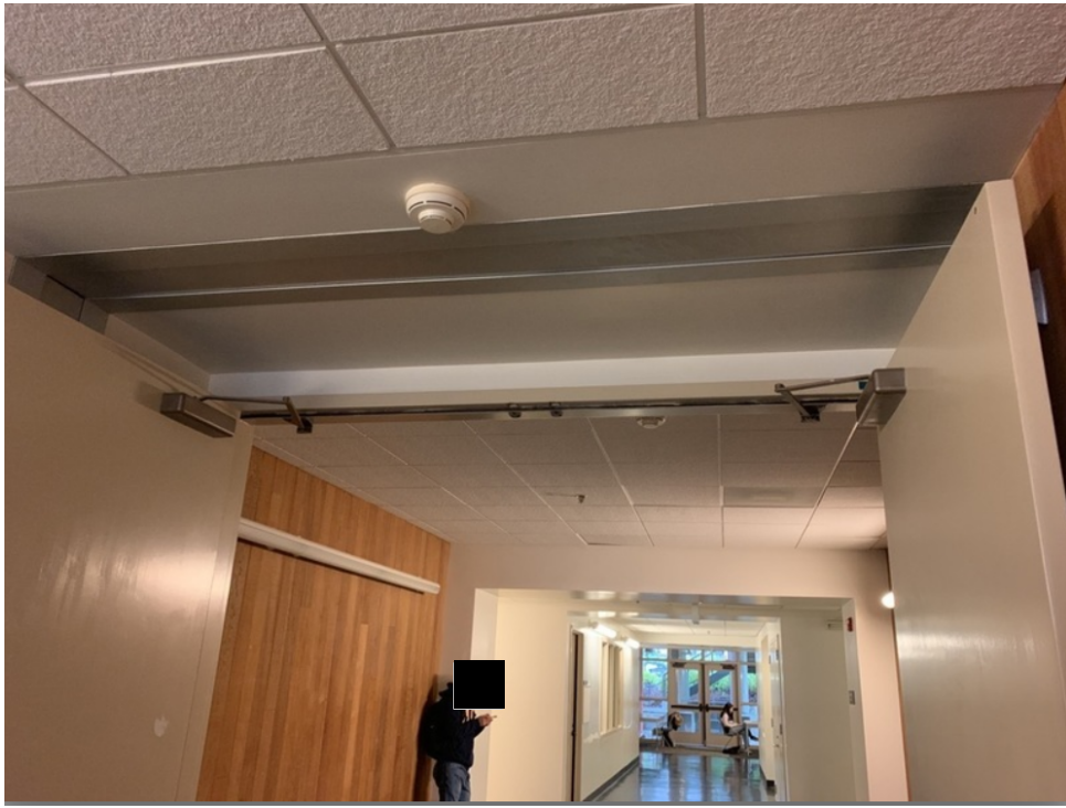
Figure 3 - View of hall way looking toward north. Seismic Joint is seen above the doors.
