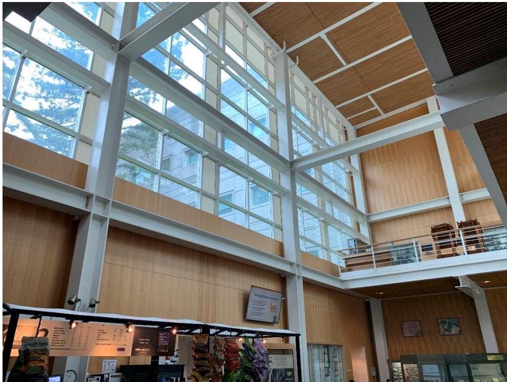
Interior View of Atrium Exposed Framing and Glazing from Café at Lowest Level of Steel Framing (Looking Southwest)
