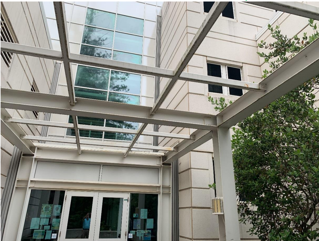
Glazing at West Atrium Entry (Looking East, Office Block A2 at Right)
