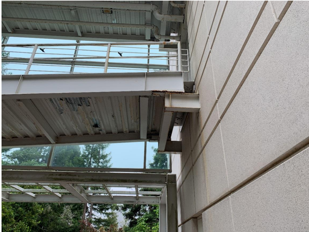
Bridge Seat (Looking South with Office Block A1 at Right, Glazing Beyond)
