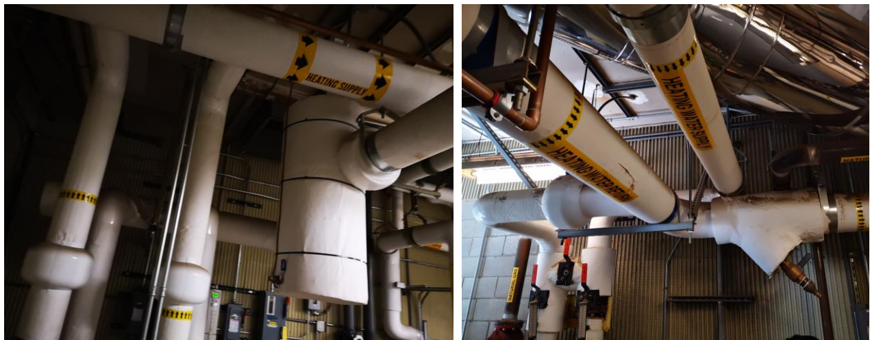
Pipes in Room 134 (cogeneration room)
