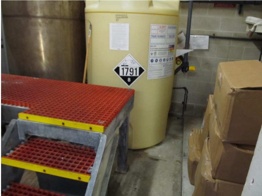
Unrestrained tank of filtration chemicals
