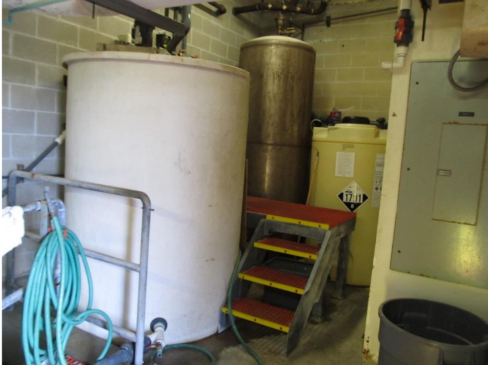
Unrestrained tanks of filtration chemicals
