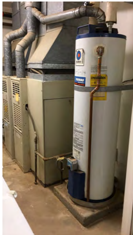
Figure 2 - MEP Equipment not anchored at base
