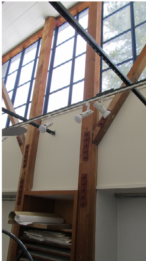
Wood Brace Frame in Enclosed Print Room (Looking Northwest; Detail K on Sheet S6)
