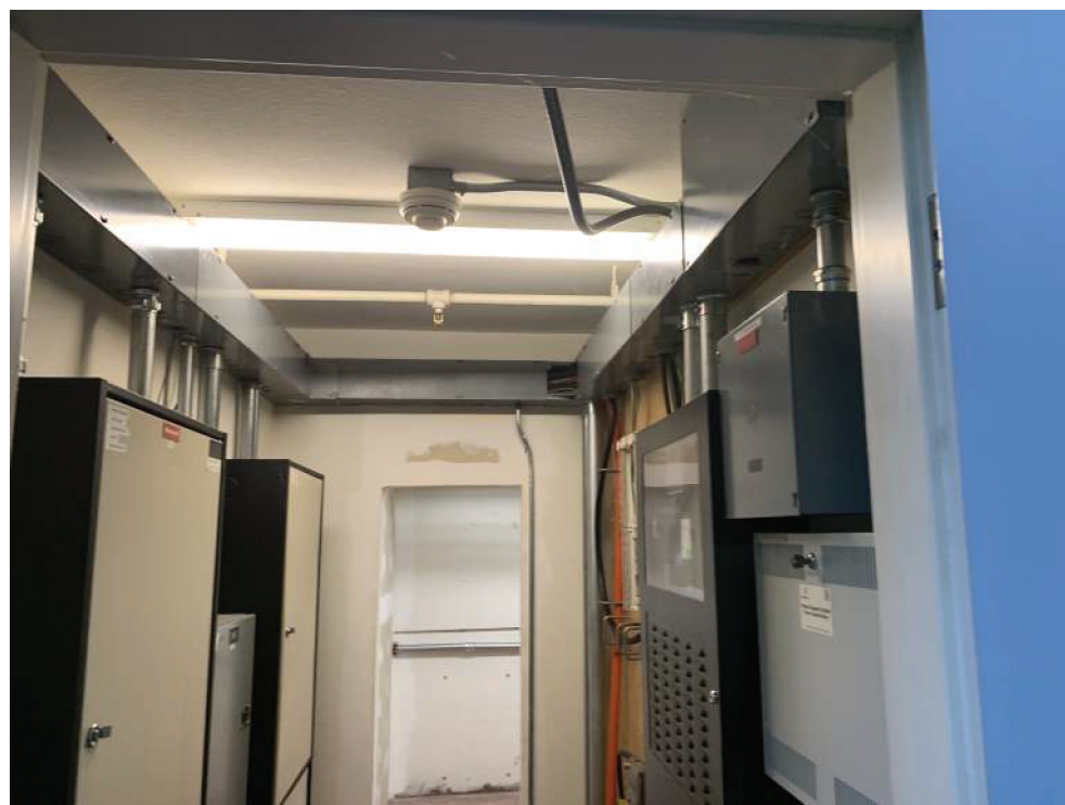
Mechanical equipment at lower floor
