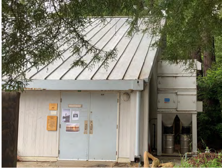
The Dust Collector near the East Wall (Looking North)
