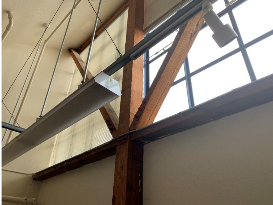
View of the South Wall at Line C from Inside Showing Truss and Clerestory Window
