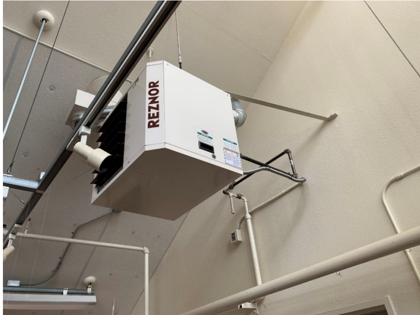
Close-up of Braced Heater
