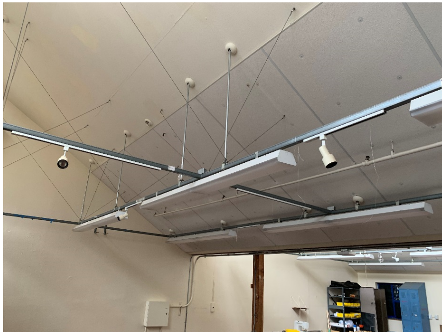
Close up of Braced Light Fixtures
