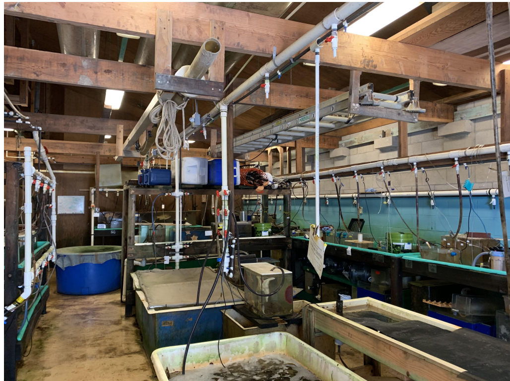
Equipment Storage Falling Hazards
