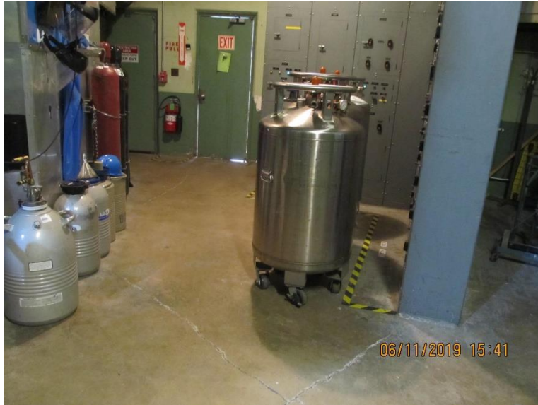
Unbraced liquid Nitrogen tanks in service area at first floor
