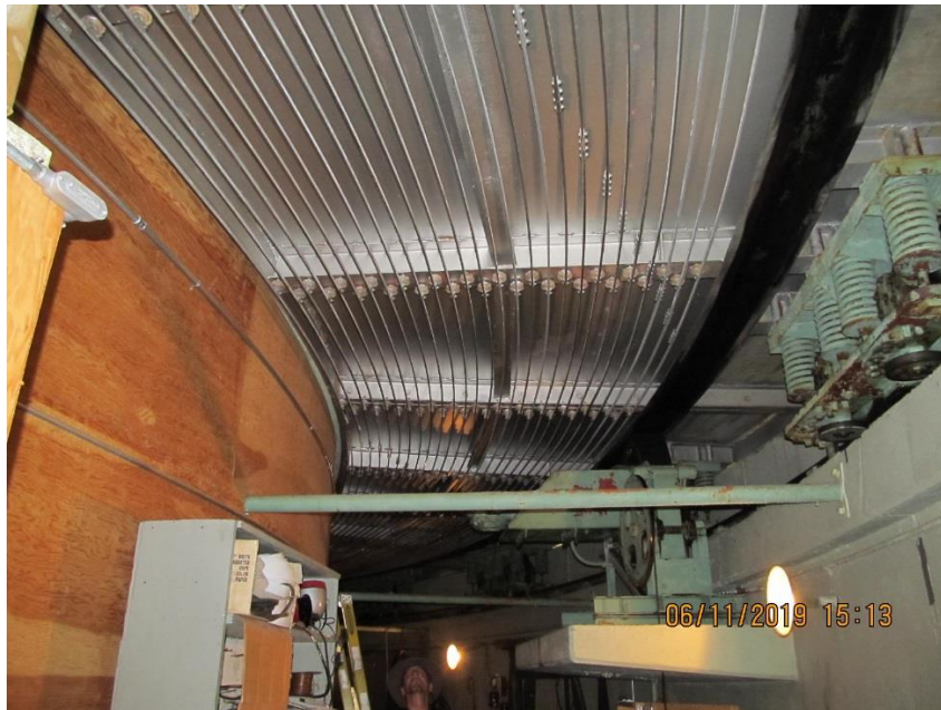
The underside of the catwalk ring with power rails that move with the catwalk/dome and are connected to fixed power supply points beyond
