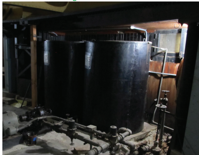
Oil Container Not Braced in the South Dome
