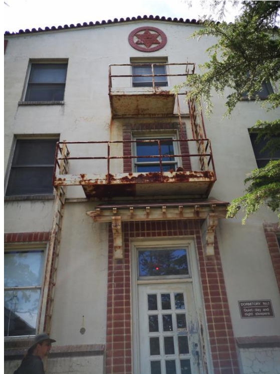
Partial East Elevation (Looking West). Note Corrosion on the East Fire Escape
