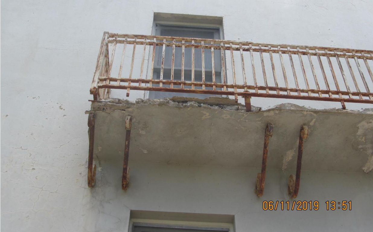
Spalling and Corrosion at North Balcony
