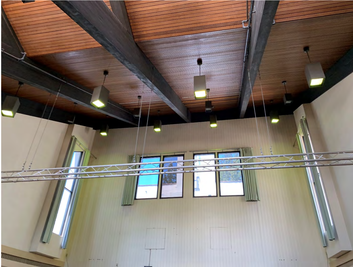
Interior view of glulam beams at high roof in Dining Hall (looking west, chimney visible through window)
