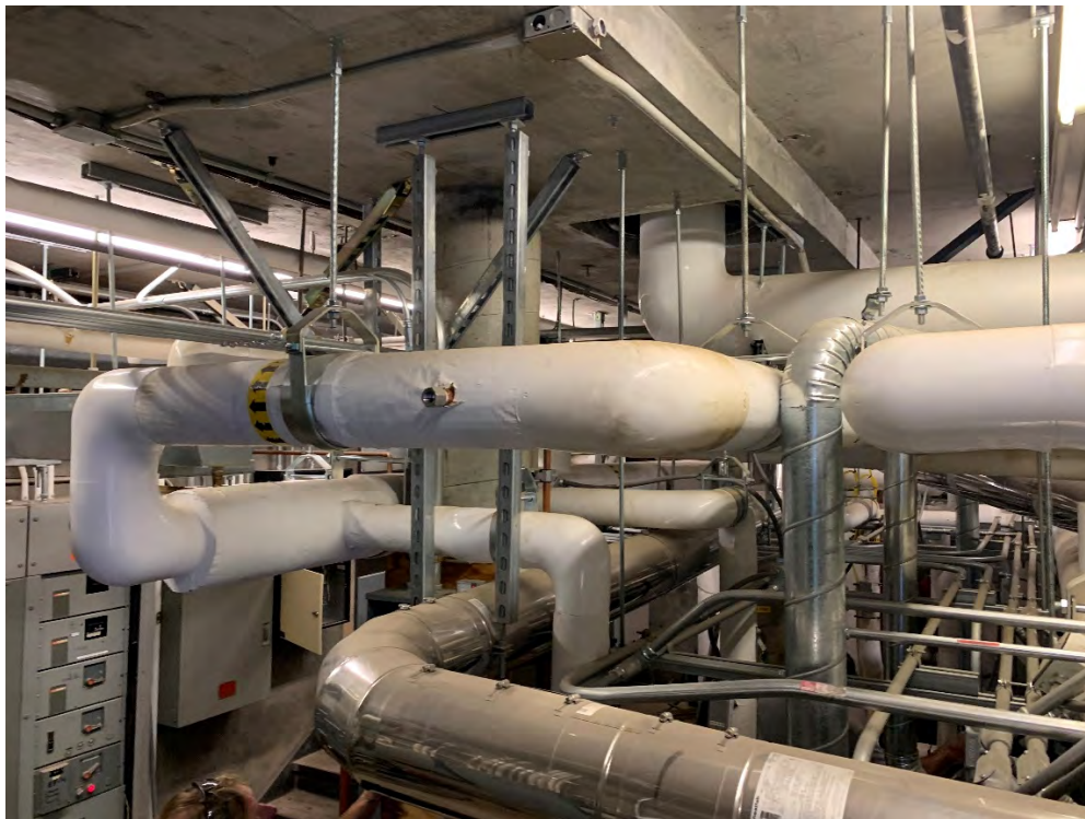
Braced piping in mechanical room at basement level below Kitchen
