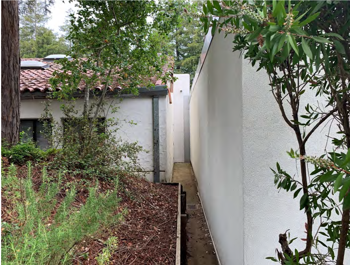
Partial south elevation showing southeast corner at rear of kitchen in center with portions of Merrill College at left and right with no visible gaps (looking north)
