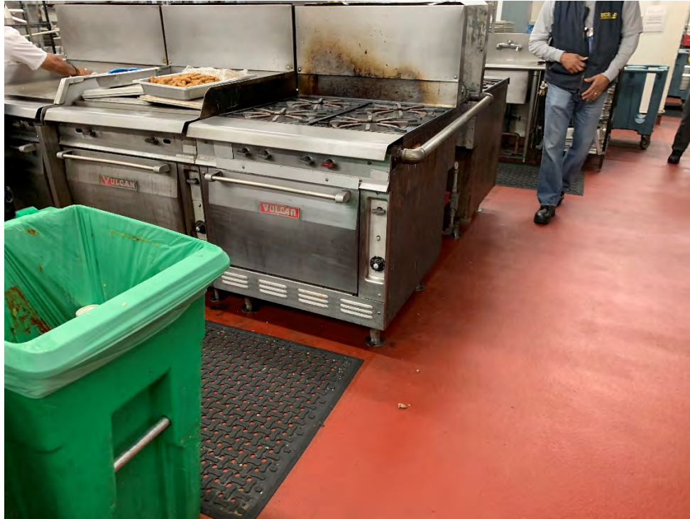
Gas-fired stoves anchored in Kitchen
