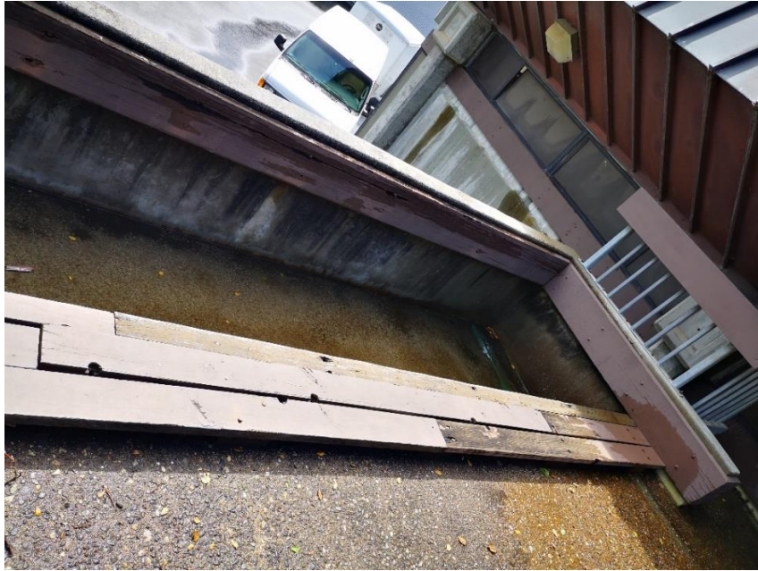
Dugout Feature along the East Edge of Roof Terrace (Looking Southeast from North Roof Terrace)
