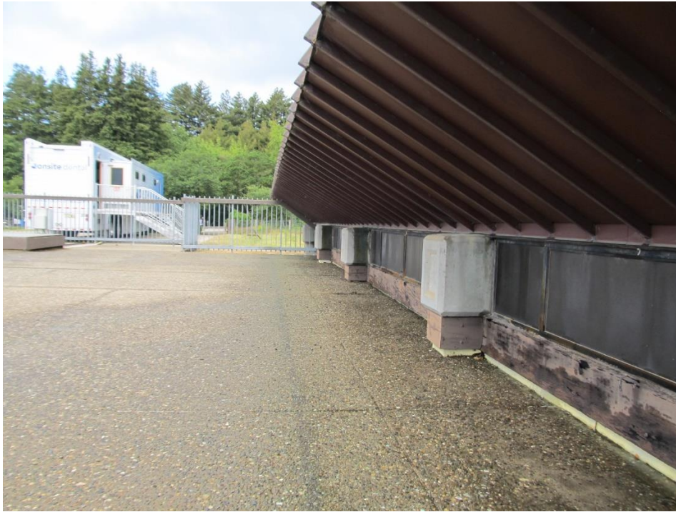
South Elevation of Clerestory Windows at General Purpose Room (Looking Southwest from South Roof Terrace)
