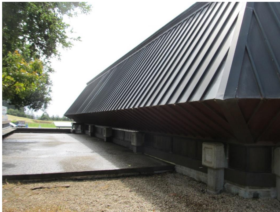
Northwest Corner of General Purpose Room (Looking Southeast on West High Grade Level)
