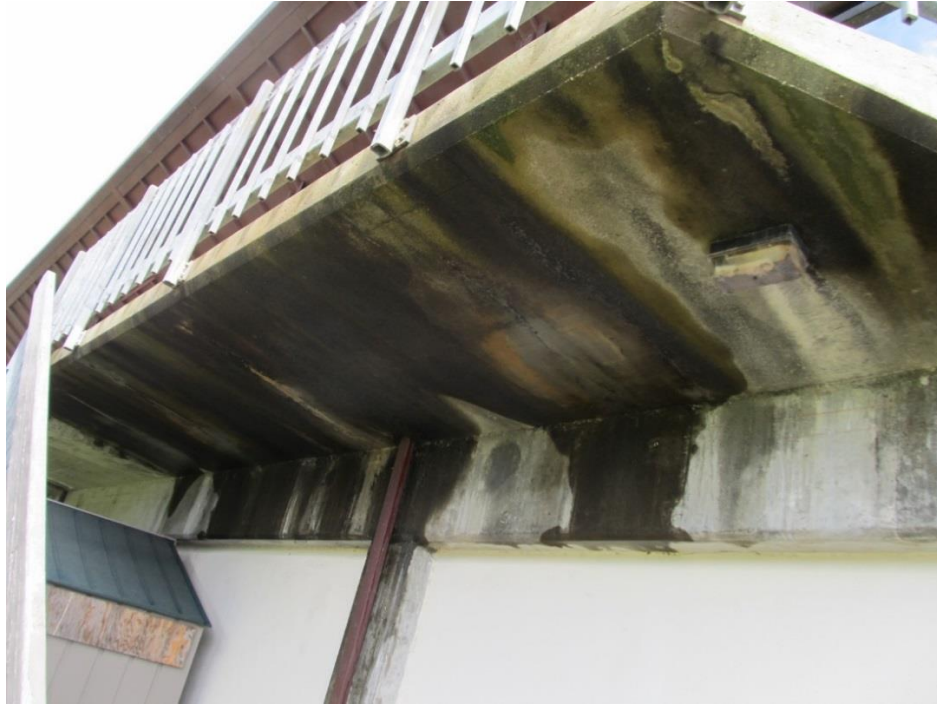
Water Marks on the Exterior Stairs Hallway (South)
